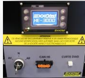
Infos, control, diagnostic
